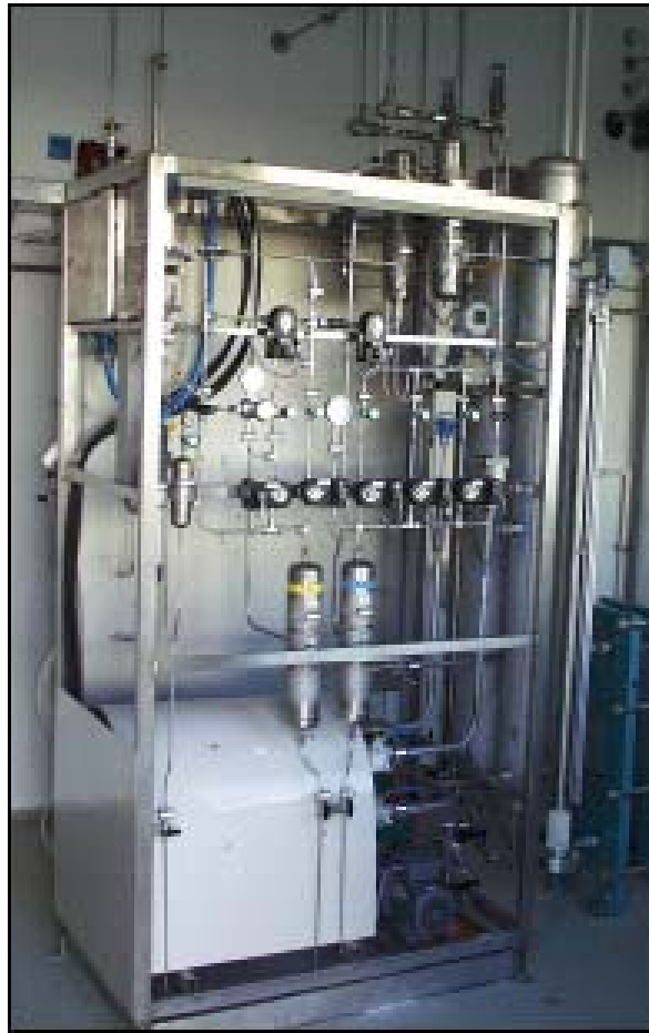
Figure 3: 20 kW pressurized electrolyser
