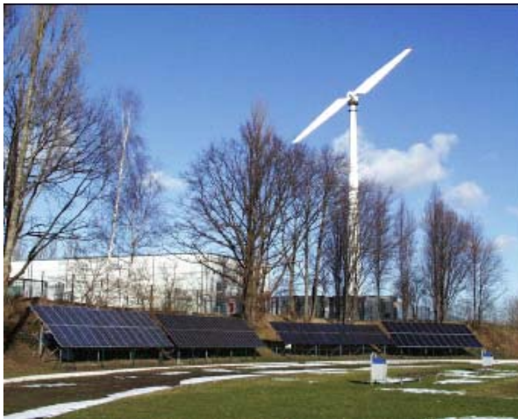
Figure 2: Photovoltaic installation and windmill
