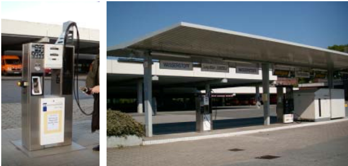
Figure 8: Hydrogen dispenser and filling station
